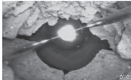
Figure 13 – Typical Crossbore Into Sewer Line
