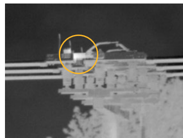
Figure 6. This third image of the substation transmission line, captured with a Fluke 4x telephoto lens clearly shows a hot spot or high resistance on a knife switch.
