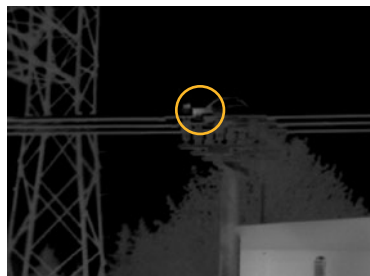
Figure 5. Scanning the same area with a Fluke 2x telephoto lens shows a definite hot spot on the switch.
