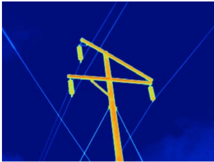
Figure 7: High voltage power pole, captured with a TiX560 camera and standard lens.
