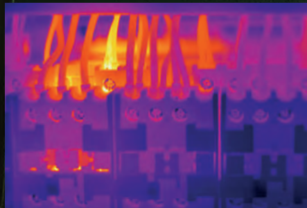
MAINTAIN SYSTEMS Identify excessively high temperatures in circuit breakers and electrical components before breakdowns occur.
