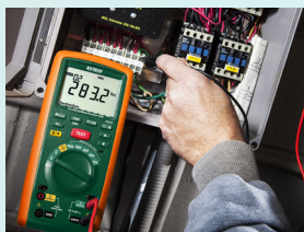
Voltage check on motor starter
