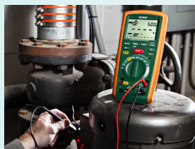
Insulation test on pump motor
