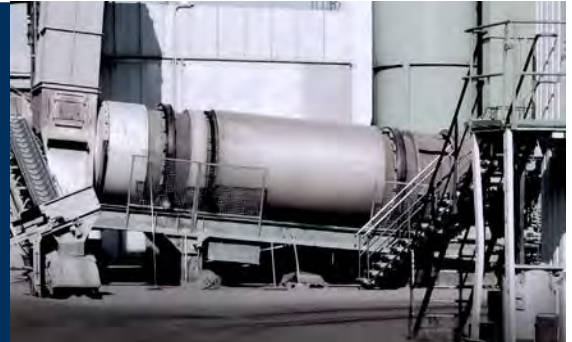
Application example: rotary kiln in the chemical industry
