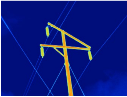
Figure 7: High voltage power pole, captured with a TiX560 camera and standard lens.
