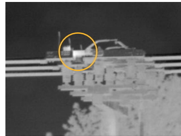
Figure 6. This third image of the substation transmission line, captured with a Fluke 4x telephoto lens clearly shows a hot spot or high resistance on a knife switch.
