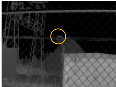
Figure 4. An exterior scan of exterior equipment at a substation with a TiX560 infrared camera and a standard lens captured an anomaly on one of the phase switches.
