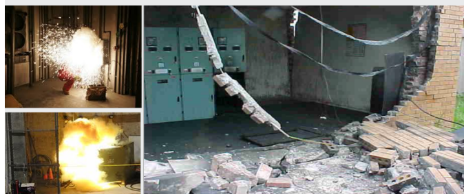
The likelihood of a shock exposure and arcing fault and arc flash increase when equipment is designed, installed, operated, or maintained improperly
